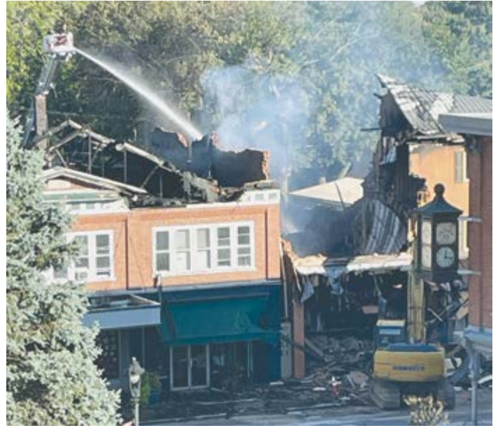
Third Street in Oxford on the afternoon of Sept. 14. Demolition had already started on what remained of the buildings gutted by the five-alarm fire.
